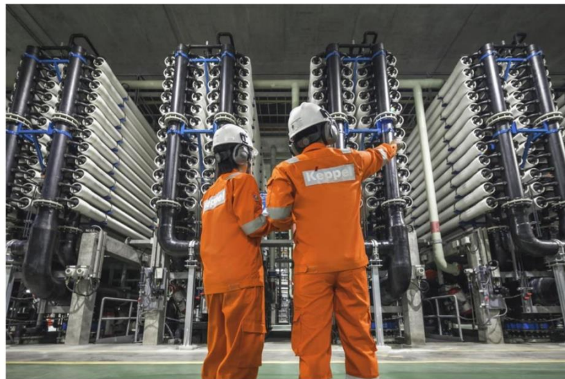
Staff at the Keppel Marina East Desalination Plant, which has an enterprise value of $323 million. PHOTO: KEPPEL CORPORATION
